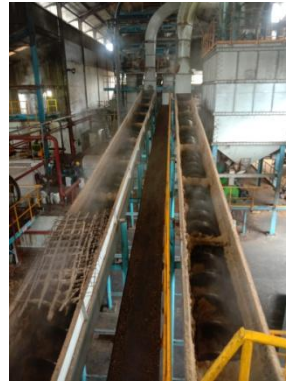
Cake Breaker Conveyor
