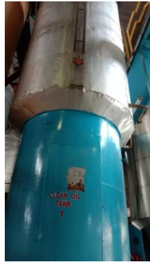
Clean Oil Tank
