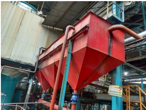
Sand Trap Tank
