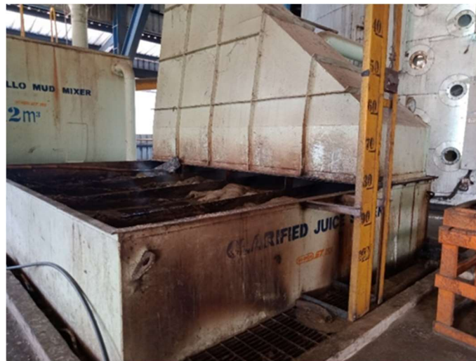
Gambar 31. Clarifier Juice Screen
