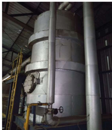
Gambar 60. Direct Contact Heater
