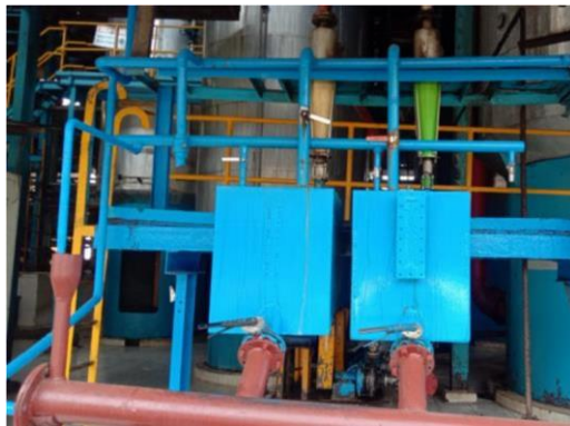
Sand Cyclone Balance Tank
