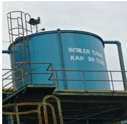
Gambar 3. 74Boiler Water Tank
