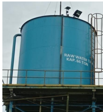
Gambar 3. 69 Raw Water Tank
