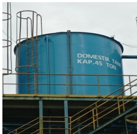
Gambar 3. 75Domestic Water Tank
