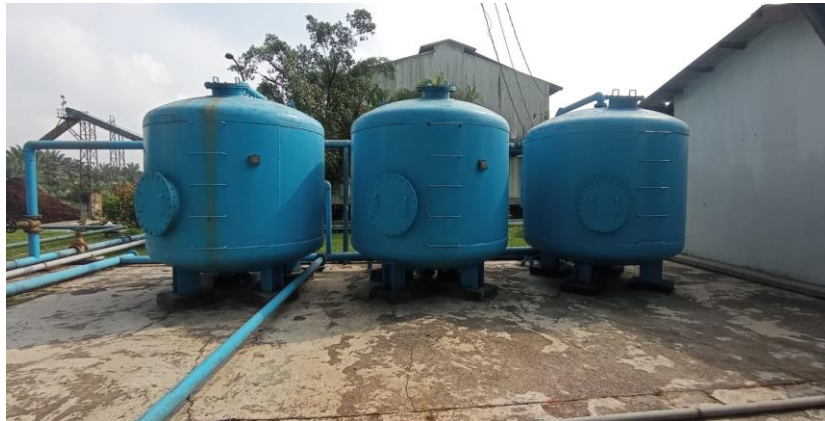
Gambar 3. 73Sand Filter Tank
