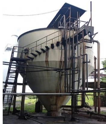
Gambar 3. 41 Oil Recovery Tank
