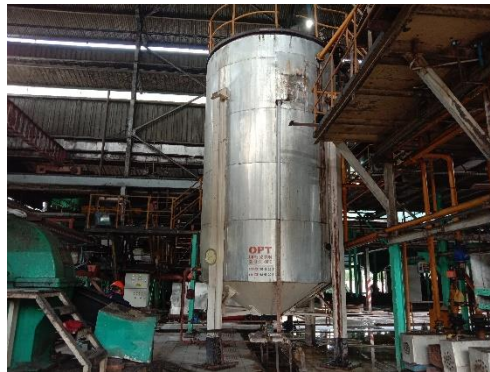
Gambar 3. 33Oil Purifier Tank
