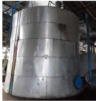
Gambar 3. 81 Feed Water Tank
