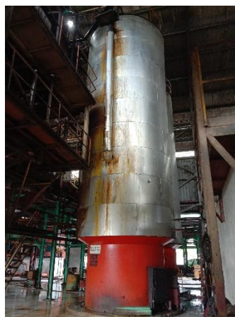
Gambar 3.32 Continous Settling Tank
