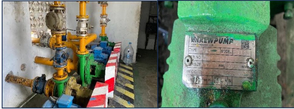
Gambar 5.7 Pompa Storage Tank
