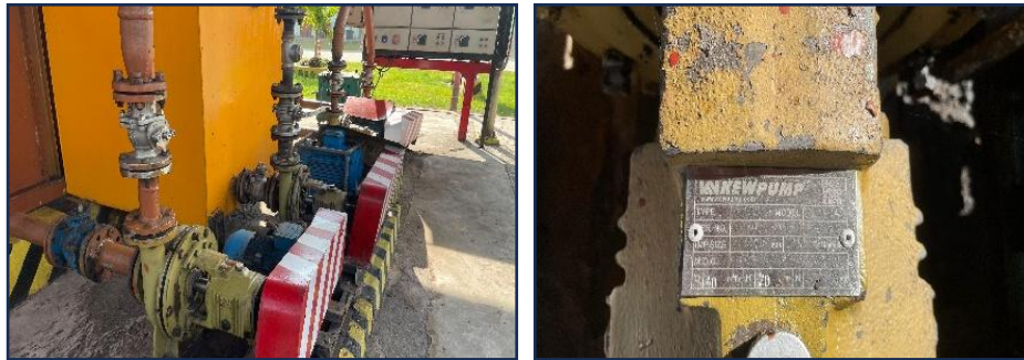
Gambar 5.9 Pompa Recovery Pit
