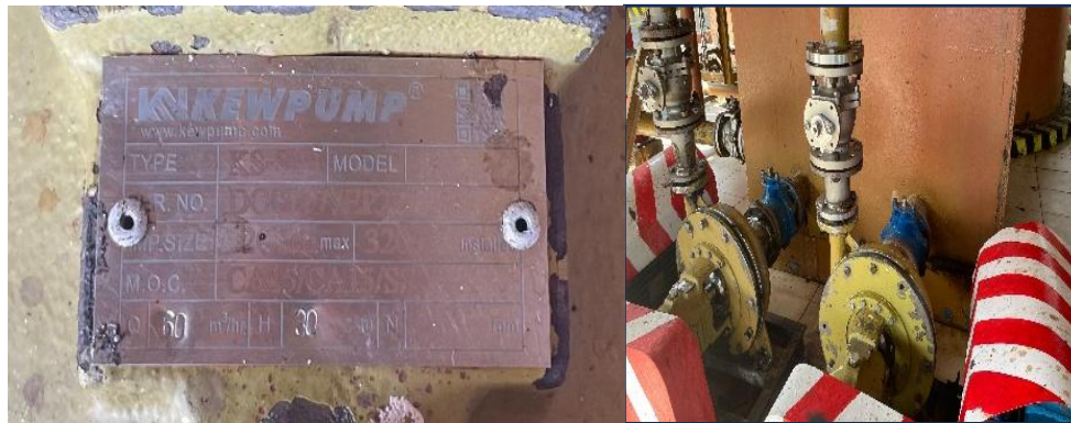
Gambar 5.4 Pompa Continuous Settling Tank
