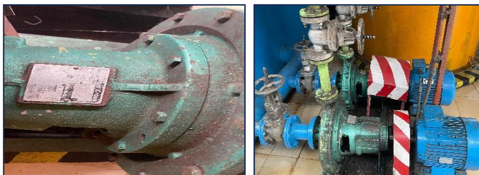
Gambar 5.5 Pompa Oil Tank
