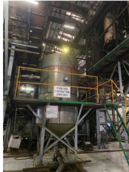
Gambar 2. 51 Sand Trap Tank
