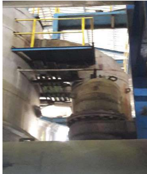
Gambar 46. Evaporation Temporary Valve
